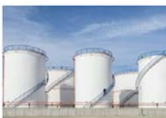
Guidance Note 52: Assessment of Customer Bulk Facilities – Revised 2020
